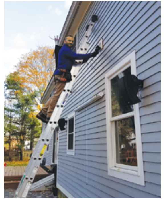
Matt Durling is pictured using an air flow meter to verify air is properly flowing without obstruction.
