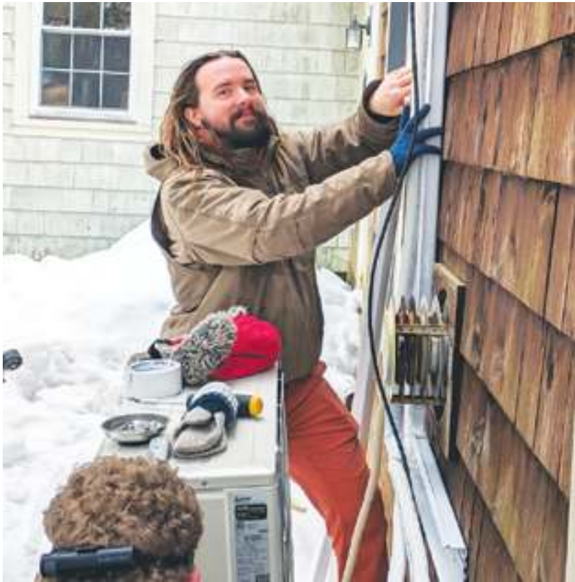
James Mayer, owner of Unity Heat Pumps, is pictured working on a recent residential installation. “We put time and care into each customer’s install to build our business and to make our world a better place,” he says.
