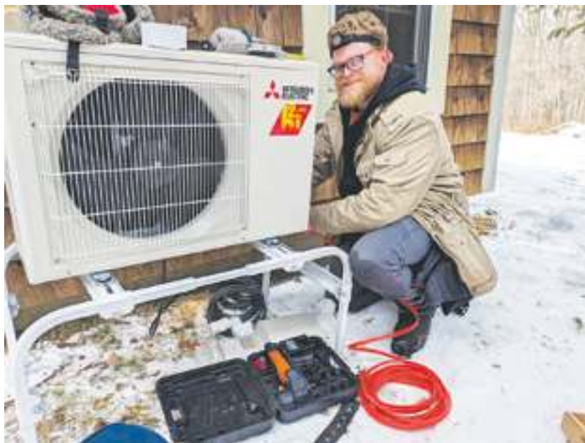
Installer Timothy Mabe is seen working on a Unity Heat Pump mini-split heating and cooling system installation.
