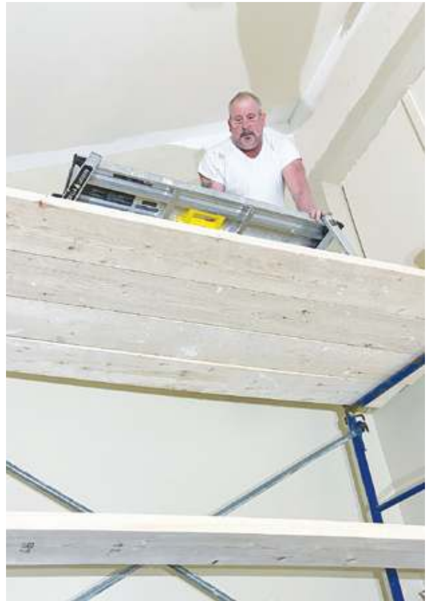
Dale Blanchard works from a scaffold on a residential project. Blanchard has been specializing in dry wall installation for more than 40 years.
