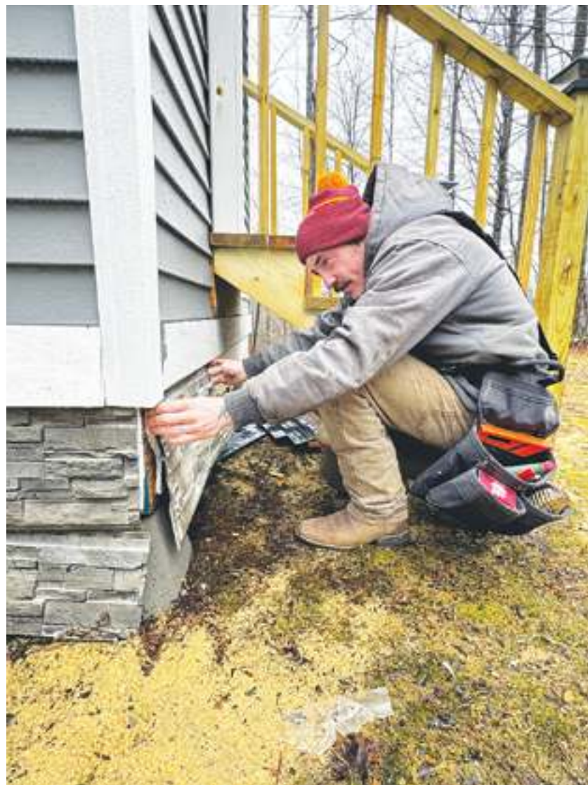
Sam Graves, employee of Elevated Home Services, is seen applying a faux-stone panel to a foundation.
