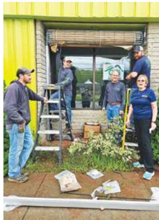
The crew at Champion Overhead Door are seen putting up security gates at the new dispensary in Brattleboro, VT. They include (L to R): Harley Banis, Ben Airher, Ed Dews, Paul Sherburn, and Janet Penfield. This local business offers expert garage door services for residential and commercial customers. For more details, call 802-251-0900 or 603-363-8800.
