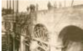
The winner of last week's Mystery Photo Contest was Joe Walier of Keene. The photo shows the power plant at the Vernon Dam during its construction in 1909.
