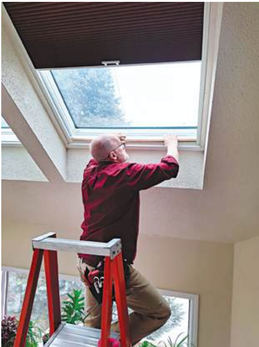
Matt DeGrosky of Monadnock Shutter & Shade is pictured installing a window treatment for a skylight. He offers both manual and motorized options.
