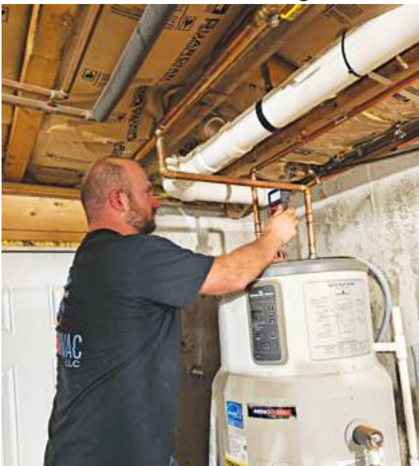
Jarrod Zieba checks the voltage on a heat pump water heater.
